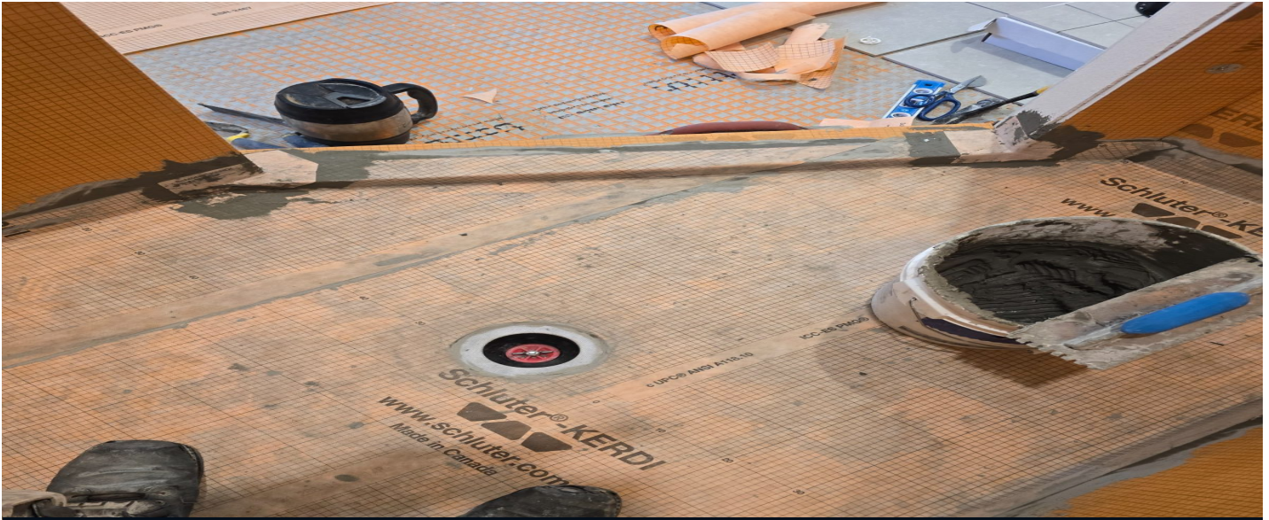
PHOTO 2 — KERDI SHOWER BASE
