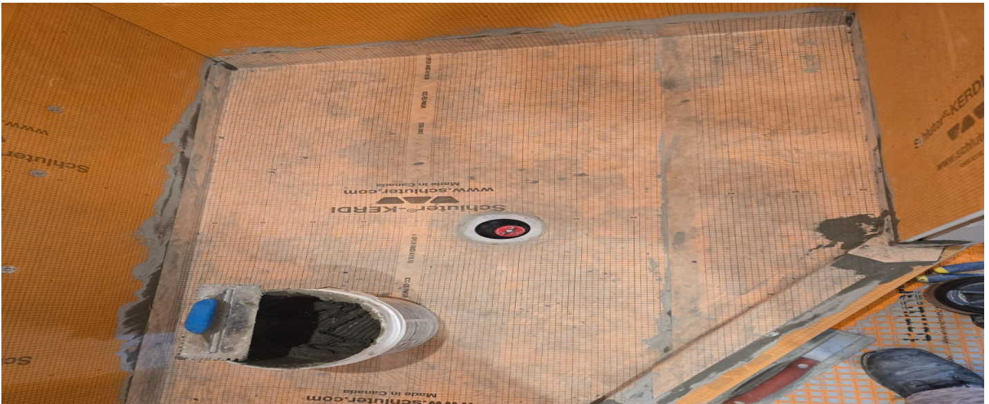
PHOTO 3 — KERDI SHOWER BASE
